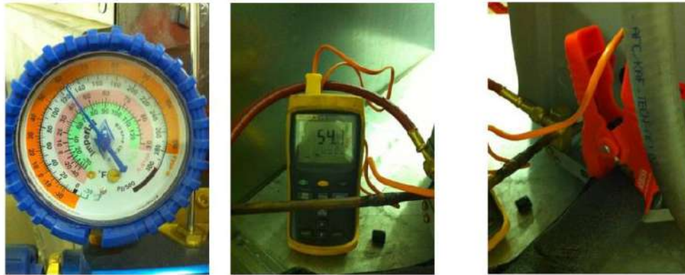
Figure 9 - Gauge Connection/Readings Suction Line
